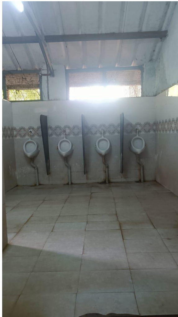
Staff wash Rooms
